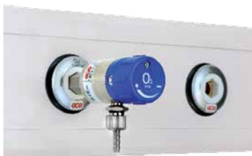
Flow selector connected to hospital terminal unit
